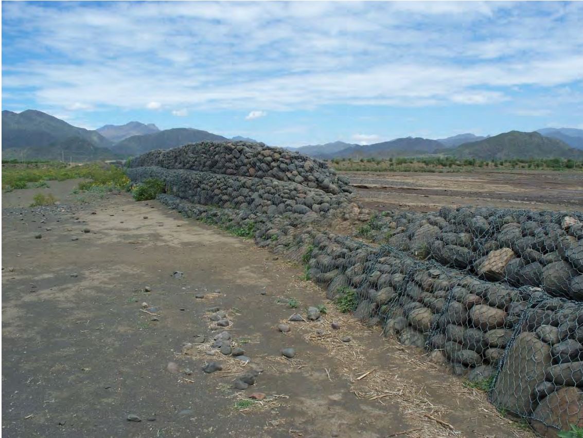
Figure 4.26 - Collapse of protection works, right bank, downstream of Highway bridge
